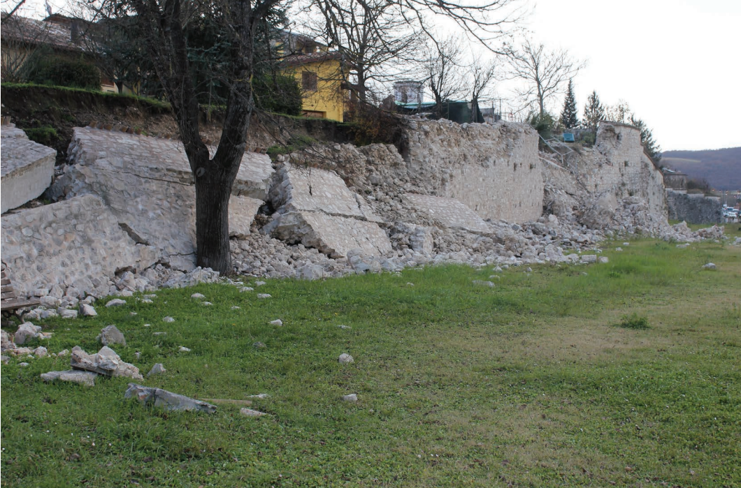
Fig. 05: Norcia, western section of the town walls after the recent earthquake.
