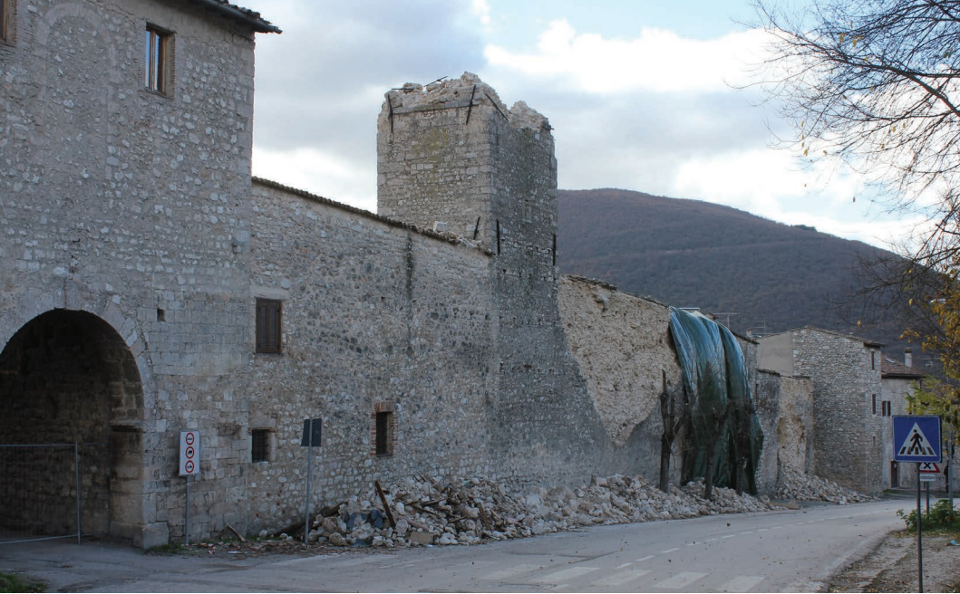
Fig. 06: Norcia, the wall near 'Porta San Giovanni', after the recent earthquake.
