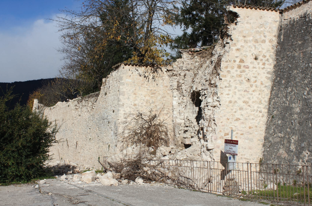
Fig. 04: Norcia, the wall near 'Porta delle Ceresce', after the recent earthquake.
